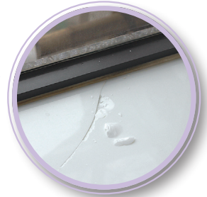
Any chipping on window hood marble slab
