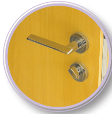
Any malfunctioning, discolouring, loosely fixed component at door locks/ handles
