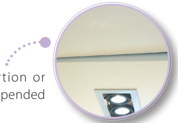
Any distortion or deformation of metal suspended ceiling
