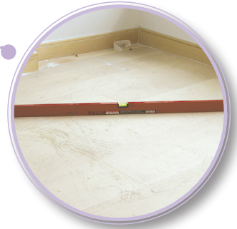
Any incorrect leveling on timber flooring
