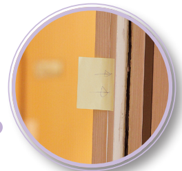
Loosen joint at door frame
