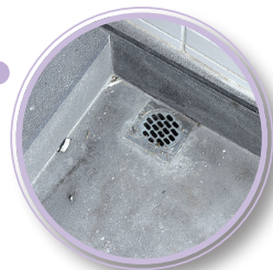
Any blockage of floor drain or corrosion of grating
