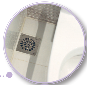
Any incorrect fall or water ponding on floor
