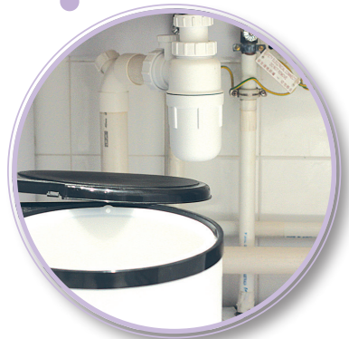
Any sign of blockage and leakage of water traps and piping connected to kitchen sink, washing machine and floor drain
