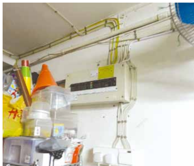
Picture 4 Difficult for the Elderly to Clean
