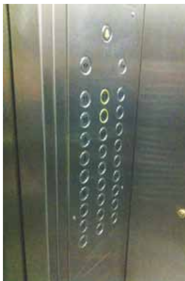
Picture 3 Too Small Lift Buttons
