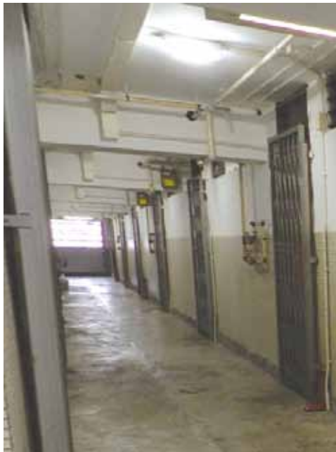
Picture 9a No Handrail in Corridor
