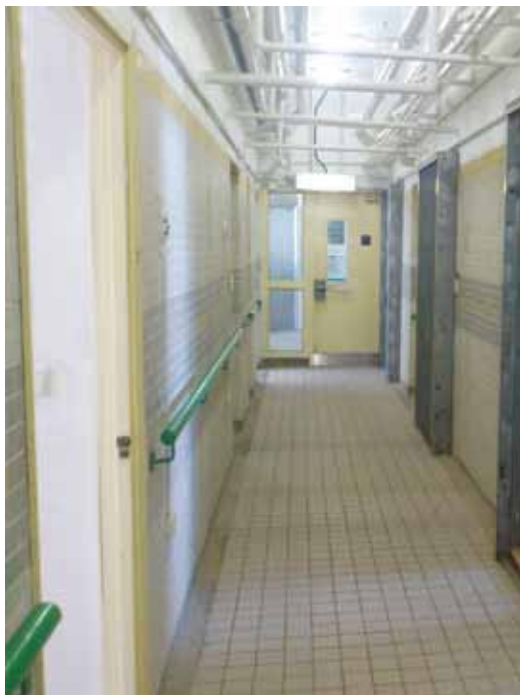
Picture 1 No Ventilation in Corridor
