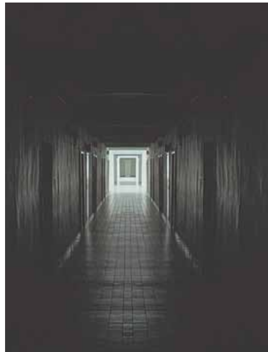
Picture 2 Poor Lighting in Corridor
