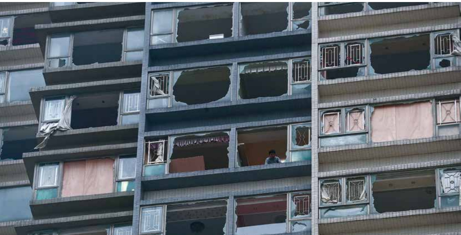
Broken windows on an apartment building in Macau, following Typhoon Hato on 23 August 2017.
