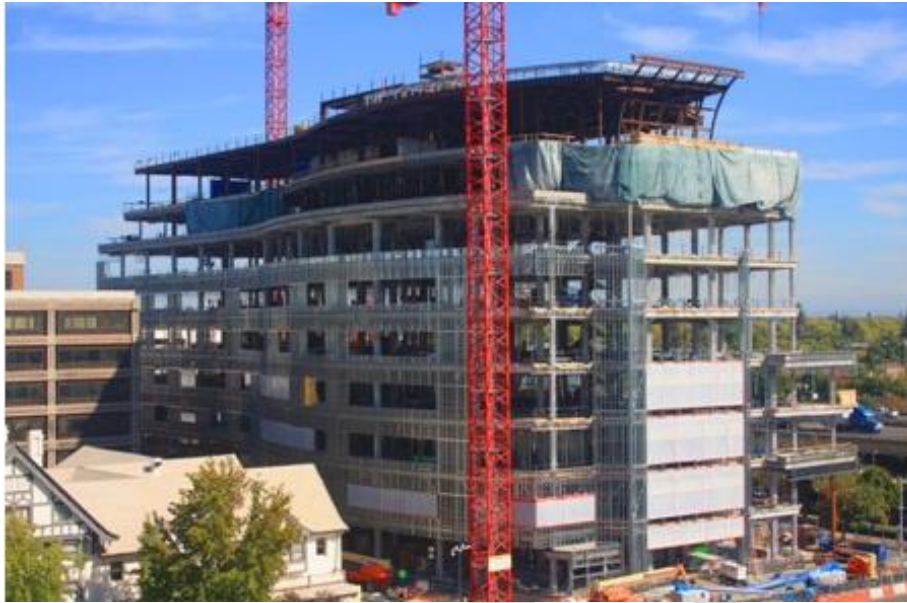
Figure 3.2. Sutter General Hospital Renovation by Turner Construction in USA (adopted from Kymmell, 2008)
