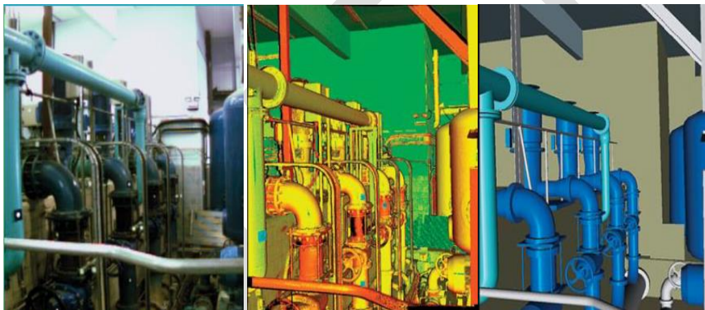
Figure 3.1. Laser Scans and resulting BIM model of a water treatment plant pump replacement (adopted from Bennett, 2009)
