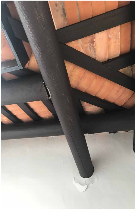
Shrinkage cracks on timber beam
