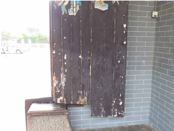
Wear and tear on timber door
