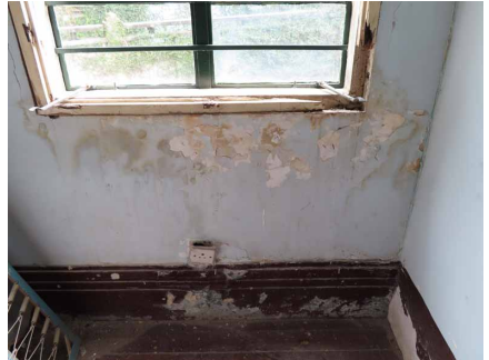
Water seepage at window surround
