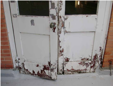
Flaking paint on timber doors
