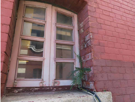
Vegetation growth on window sill
