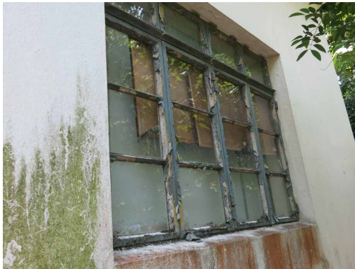
Flaking paint on metal window frame
