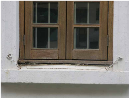
Gaps at window surround
