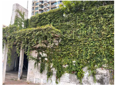
Climbing plants including diverse-leaved creeper and creeping fig growing on the vertical surface of a building
