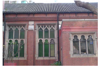
Windows with carved granite framing in the form of trefoil-headed tracery, Kowloon Union Church at Yau Ma Tei
