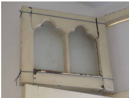
Dislodged timber frame on top vent
