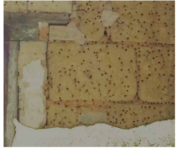
Pitting on mud bricks by insects will increase the risk of water penetration.
