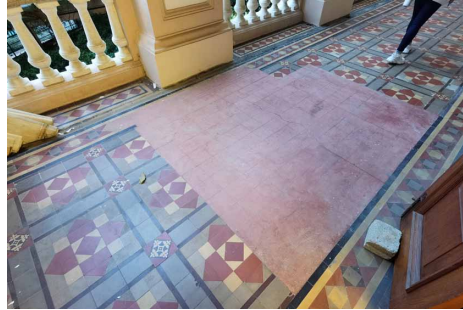
Damaged tiles were replaced by improper tiles
