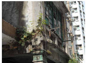
Fern and small trees growing on the vertical surface of the building. Moss stains can also be found.
