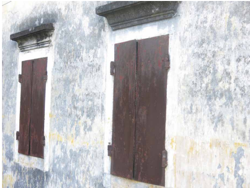
Flaking paint on metal windows
