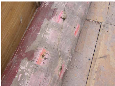
Mud tube on timber purlin
