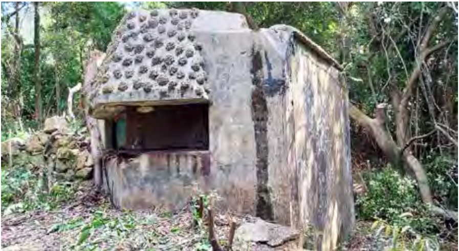
Figure 26: Exterior left side view of OP Middle Gap showing remains of squatter improvisations (1 November 2021 by Lawrence W.C. Lai)
