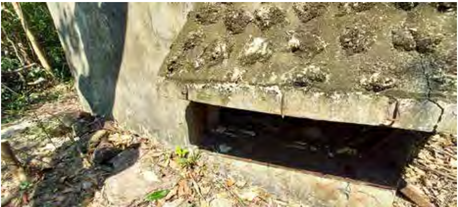
Figure 57: Metallic hooks, like those on the OP Middle Gap, on one of the apertures of OP Middle Spur
