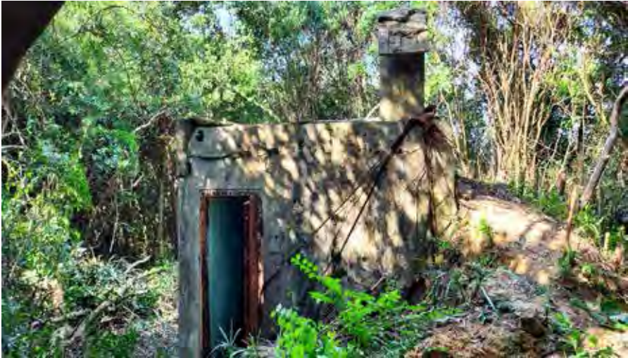
Figure 27: Exterior rear view of OP Middle Gap showing the entrance, with its steel door wide open, and ventilation shaft (1 November 2021 by Lawrence W.C. Lai)
