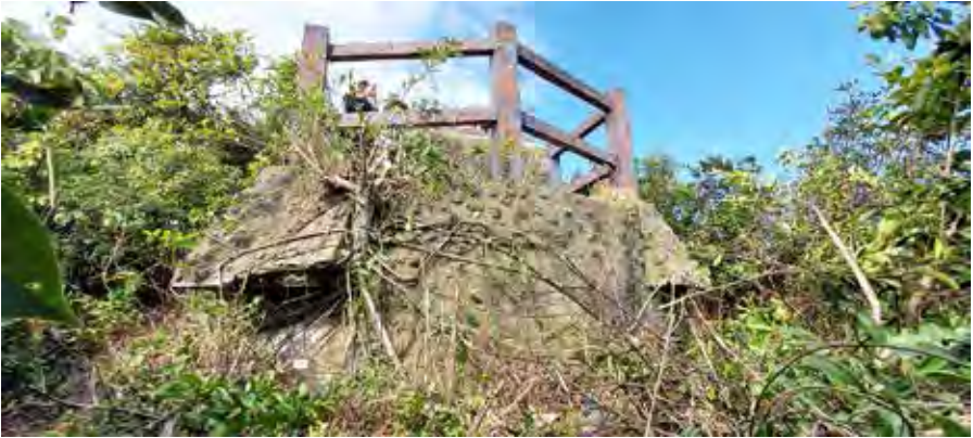
Figure 1: Exterior front view of OP Stanley Mound (17 February 2021 by Lawrence W.C. Lai)
