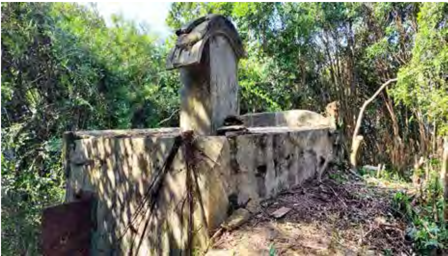
Figure 28: Exterior rear side view of OP Middle Gap showing the entrance, with its steel door wide open, ventilation shaft, and apex (1 November 2021 by Lawrence W.C. Lai)
