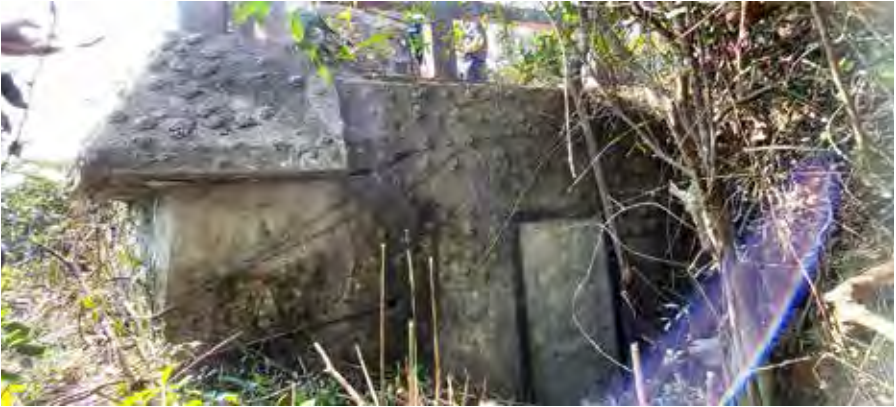
Figure 3: Left side view of OP Stanley Mound showing the entrance and left aperture blocked by concrete (17 February 2021 by Lawrence W.C. Lai)
