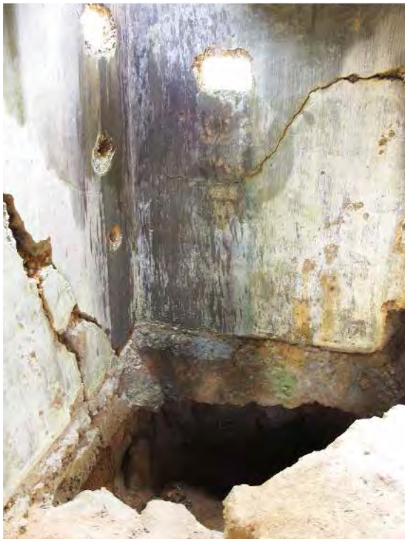
Figure 18: A tunnel portal within OP Braemar Hill (27 December 2021 by Lawrence W.C. Lai)
