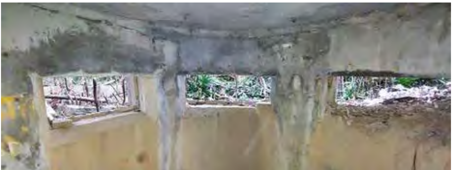
Figure 7: The three embrasures seen from within the structure (8 February 2022 by Lawrence W. C. Lai)
