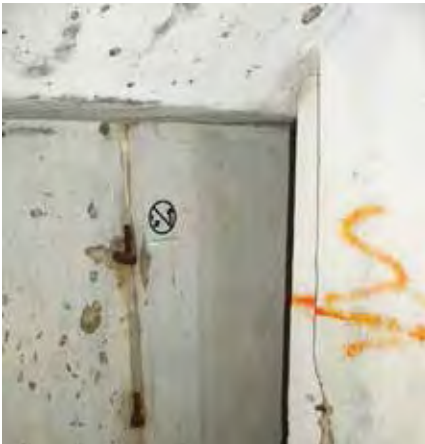
Figure 6: Doorway at top of staircase connecting the OP and the kitchen of SMR, showing remaining hinges (Taken by Y.K. Tan)
