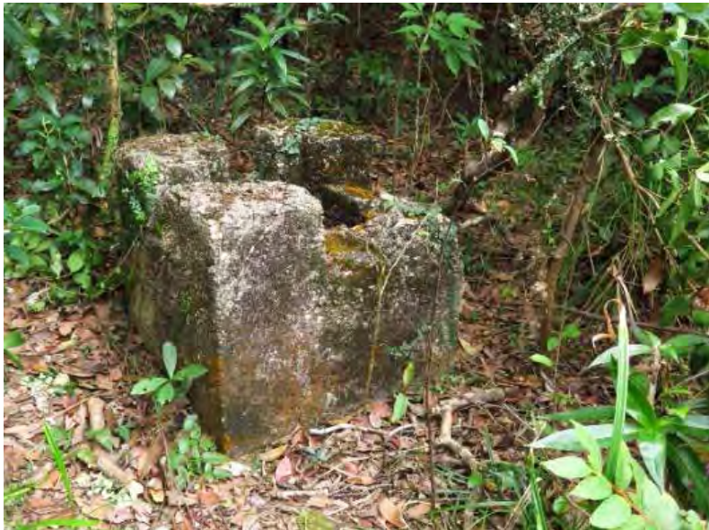
Figure 4: Ventilation opening on roof OP Shaukeiwan (Shau Ki Wan) (31 December 2021 by Lawrence W.C. Lai)
