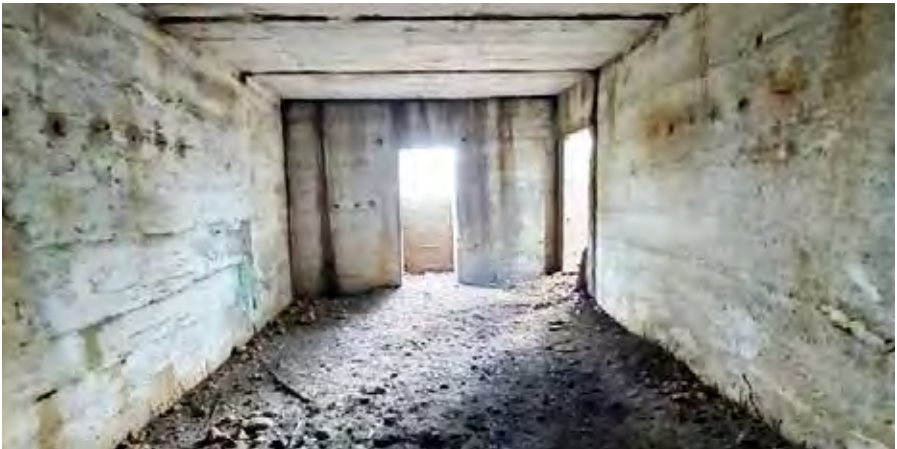
Figure 8: Interior view of OP Shaukeiwan (Shau Ki Wan): note the exposed parts of the steel frames supporting the roofs and the ‘door’ opening to the observation point (31 December 2021 by Lawrence W.C. Lai)
