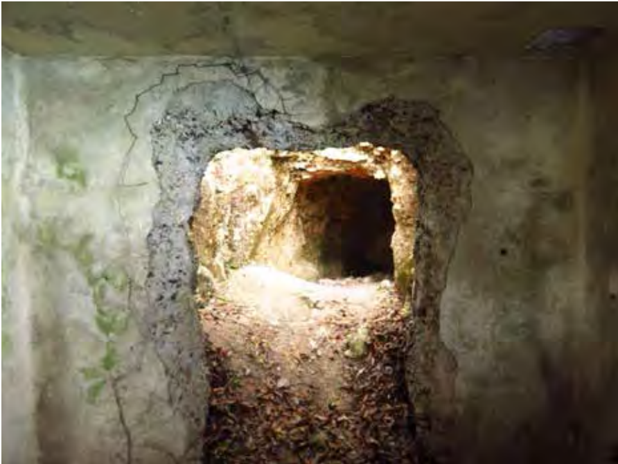
Figure 51: An earth tunnel portal behind the punctured rear wall of OP Matilda (31 January 2022 by Lawrence W.C. Lai)
