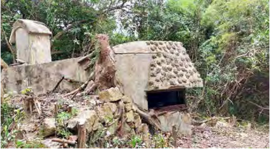
Figure 25: Exterior right side view of OP Middle Gap showing a more or less intact ventilation shaft (9 November 2021 by Lawrence W.C. Lai)
