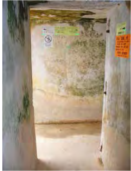
Figure 7: Exit from the kitchen of the SMR showing the remaining marks of the hinges of the door to T3 and the tunnel to Charing Cross (Taken by Y.K. Tan)
