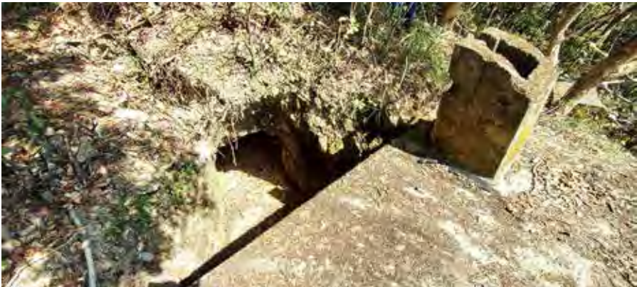
Figure 47: Rear roof of OP Matilda with its damaged ventilation shaft & portal of an earth tunnel behind (1 February 2021 by Lawrence W.C. Lai)
