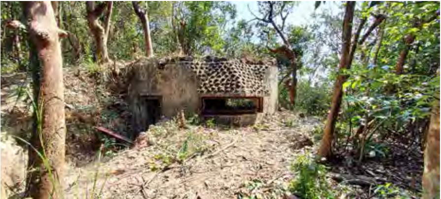
Figure 55: Exterior side view showing the entrance of OP Middle Spur (17 February 2021 by Lawrence W.C. Lai)
