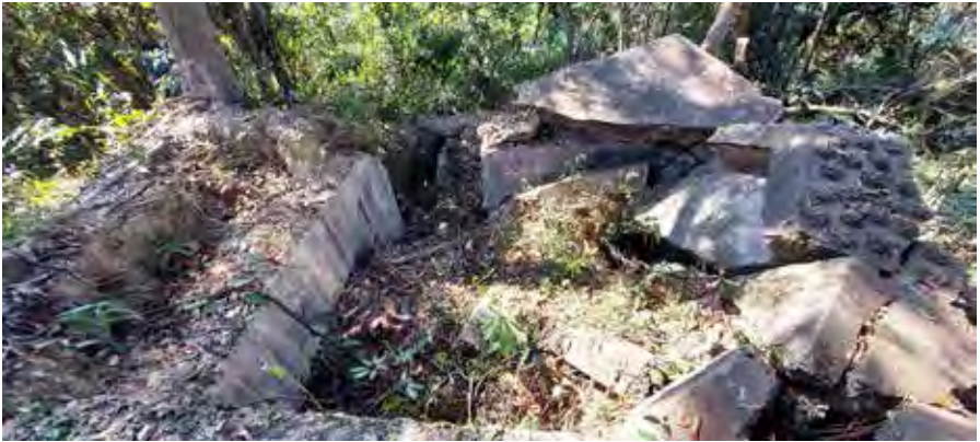
Figure 34: Top view from rear of OP Wanchai Gap (3 February 2021 by Lawrence W.C. Lai)
