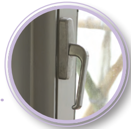
Any signs of oxidized/ corroded door handle and lock
