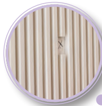
Missing door viewer
