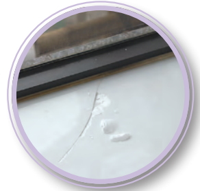
Any chipping on window hood marble slab
