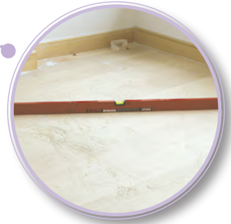
Any incorrect leveling on timber flooring
