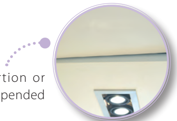
Any distortion or deformation of metal suspended ceiling
